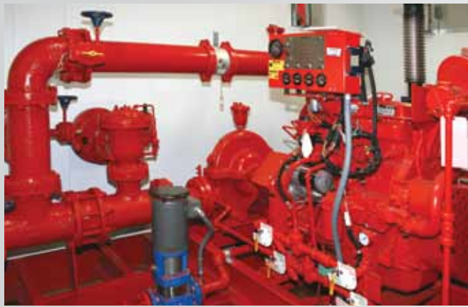
Typical housed diesel driven fire pump with test meter.
