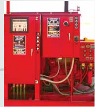
Controllers mounted and wired on diesel pump base.
