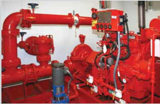
Typical housed diesel driven fire pump with test meter.
